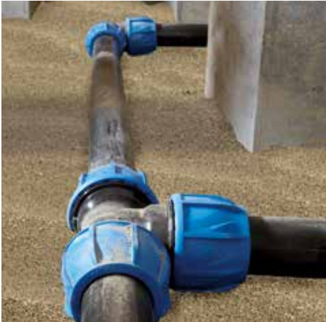
Water Distribution Lines
